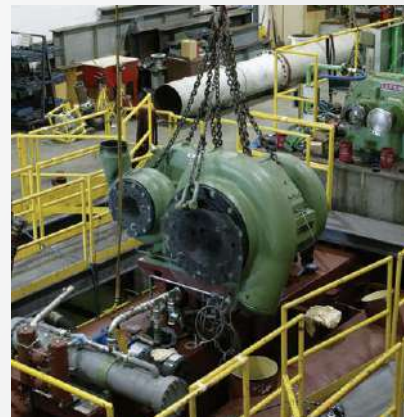
Multi-stage carbon monoxide compressor being prepared for closed-loop testing
